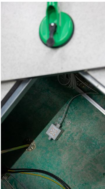
Kentix leakage sensor in raised floor
