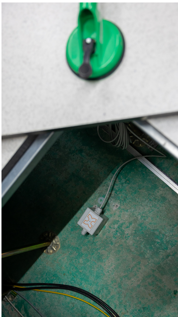
Kentix leakage sensor in raised floor
