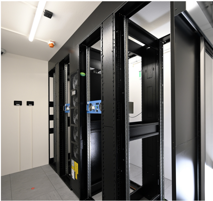
MultiSensor-TI in the Fix Container server room
