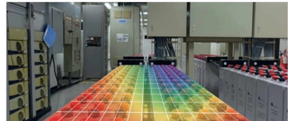
Battery UPS systems
